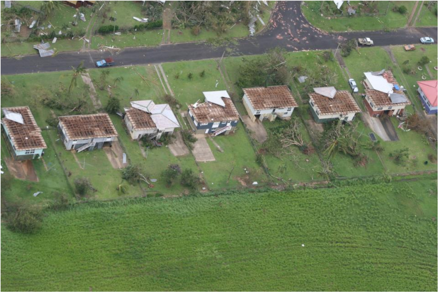
Cyclone damage in Queensland, 2009
