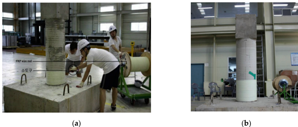
Figure 6. GFRP wire jacking: (a) Winding of the GFRP wire; (b) completed GFRP winding [58-Elsevier Copyrights].
