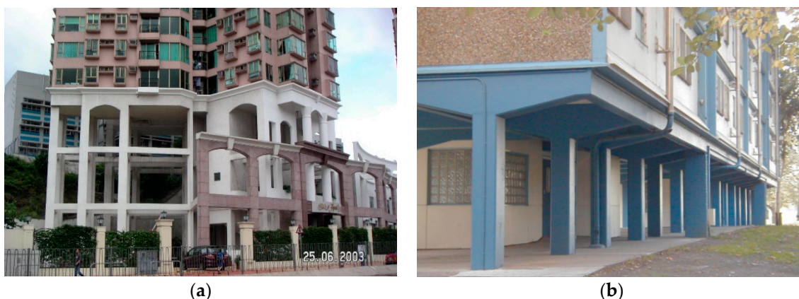
Figure 6. Potentially vulnerable beam-column connections in an earthquake: (a) High-rise residential building in Hong Kong with irregular floor plan supported by reinforced concrete frame below a transfer plate structure; (b) low-to-medium-rise residential building in Melbourne supported by precast reinforced concrete columns at the ground floor forming soft- and weak-storey (photos were taken by the author).
