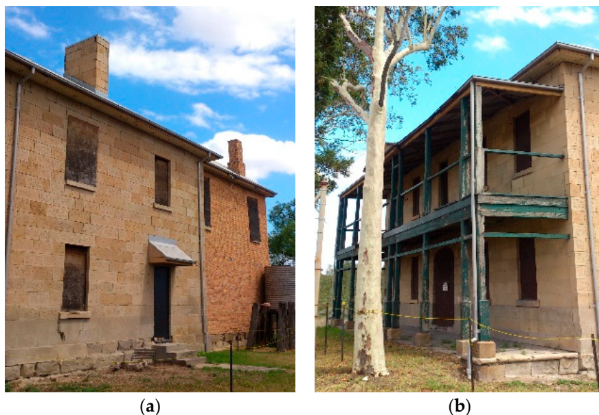
Figure 3. Damaged heritage buildings in Liddell, NSW, Australia: (a) Ashlar stone and sandstock brickwork constructions; (b) damaged timber verandah columns and supporting beams (photos were taken by the author).
