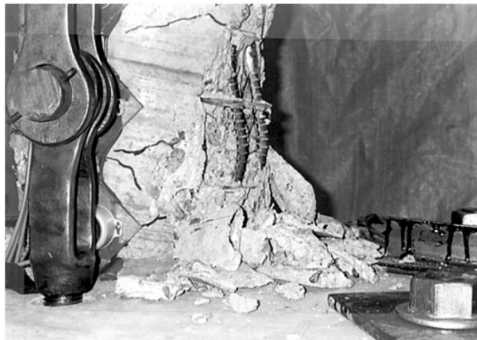
Figure 5-7. Failure of pier specimen C-2 (Saadatmanesh et al., 1997).
