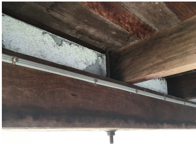
FIGURE 4 CYCLONE RODS OF EXISTING STRUCTURE AT EVERY 2 ND TO 3 RD RAFTER SPACING
