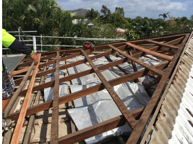
FIGURE 1 REROOF IN PROGRESS, ORIGINAL ROOF CLADDING REMOVED, NEWLY ADDD SOFTWOOD BATTENS CAN BE SEEN AND COROSION OF EXISTING ROOF CLADDING OBSERVED
