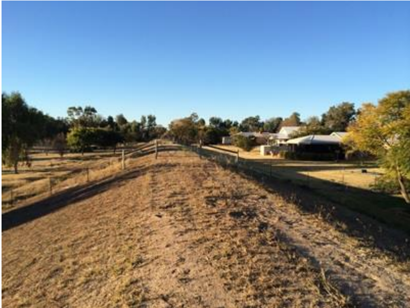
Figure 4: Flood levee constructed by the Balonne Shire Council (Okada, 10 August 2014) The major mitigation measure protects a large part of the town. Some sections of the levee have a height of several metres going through private properties.
