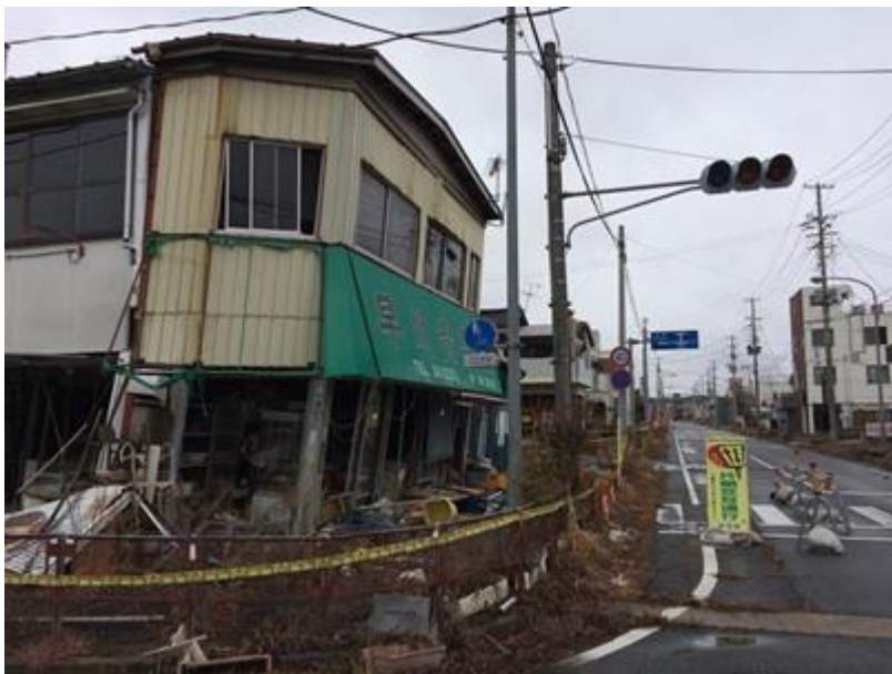
Figure 18: Unrepaired damage in Central Namie (Okada, 19 February 2015) Many buildings were left unfixed in the Town. No one lives in Namie Town (as of November 2016), because the town's entire 21,000 residents are still under the evacuation order.
