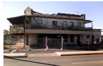
Images top-bottom: York Town Hall; Earthquake damage to Boulder heritage building from 2010 Kalgoorlie earthquake; Earthquake damage to Boulder Hotel from 2010 Kalgoorlie earthquake.
