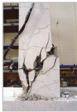
Before axial load failure
