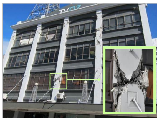
Figure 3-8: Column shear failure of a 4-storey RC frame-wall building during Christchurch earthquake in 2011 (Kam et al., 2011)
