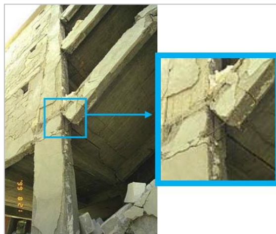
Figure 3-5: Slip of bottom beam bars due to poor embedment of bars in the joint region (Sezen et al., 2000)
