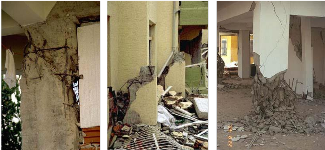
Figure 3-9: Damage experienced at the end of columns during the Kocaeli (Turkey) earthquake in 1999 (Sezen et al., 2000)
