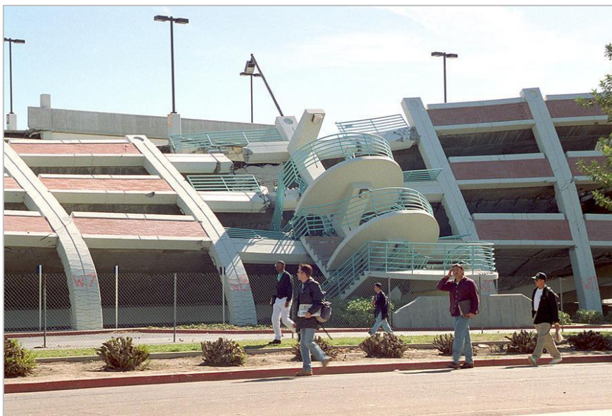
Figure 3-19: Photograph of the carpark at the California State University Northridge Campus taken after the 1994 Northridge (The Atlantic Monthly Group, 2014)
