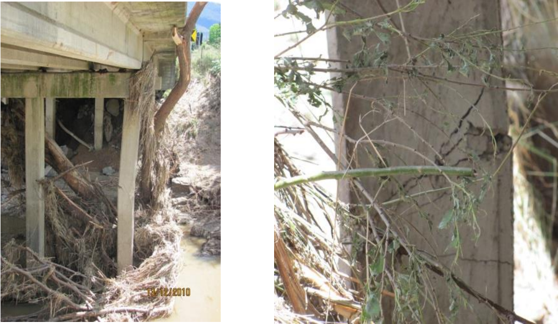
Figure 5-1: Damaged U-Slab Bridge under log impact during flooding, Victoria, 2010
