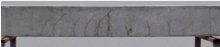
Figure 4-6: Crack propagation in the RC beam for the drop height of 0.3 m, the mass of 400 kg (Fujikake et al. 2009)
