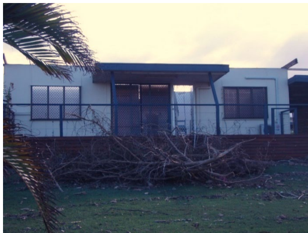
FIGURE 2 DAMAGE TO A HOUSE DURING TC LARRY
