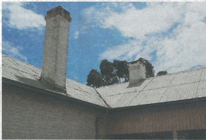
above: Two chimneys at the Residency Museum, York; image courtesy Quoin Consulting Heritage Engineers
