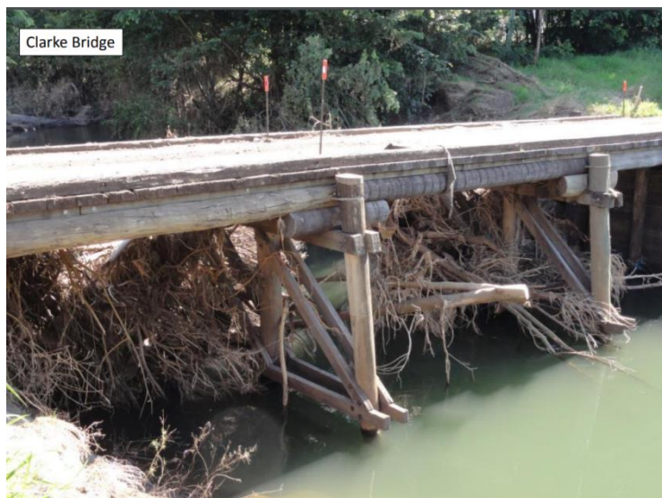
Figure 7-3 The damaged Clarke Bridge after the 2011 floods
