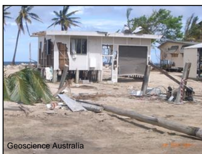
Storm surge damage from Cyclone Yasi, Tully Heads, February 2011
