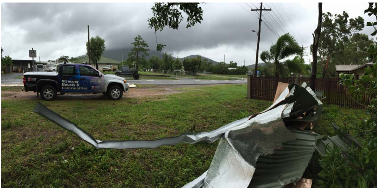
Figure 18. Metal roof cladding removed from wind uplift and blown across street (Note: cladding from the structure in the previous figure)
