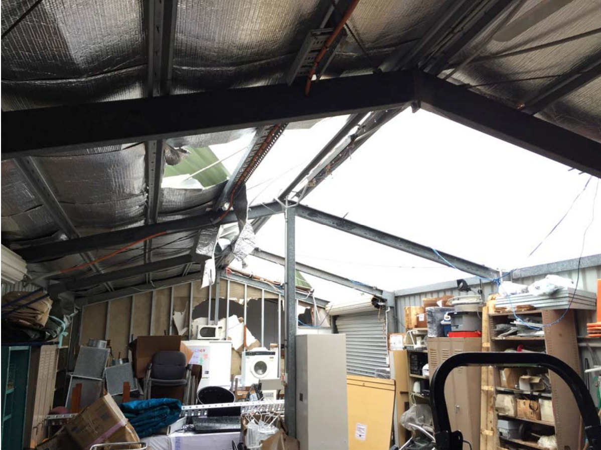
Figure 17. Interior view of metal roof cladding damage to portal structure (see Figure 16)
