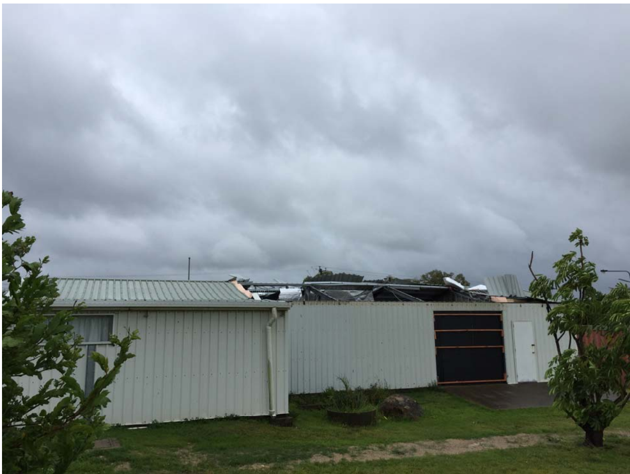
Figure 16. Wind damage to metal roof cladding and battens in Cooktown (Note: roller door was damaged during TC Nathan approach to coast in previous week)
