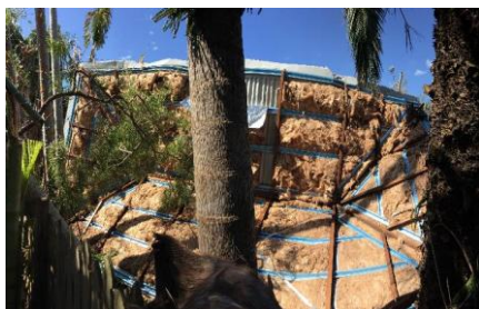
Wind-induced failure of a new (< 1 year) metal cladding roof on an old house at the rafter to top-plate connection during Cyclone Marcia (2015) in Yeppoon, Australia - there appeared to be no retrofitting of the weaker connections.
