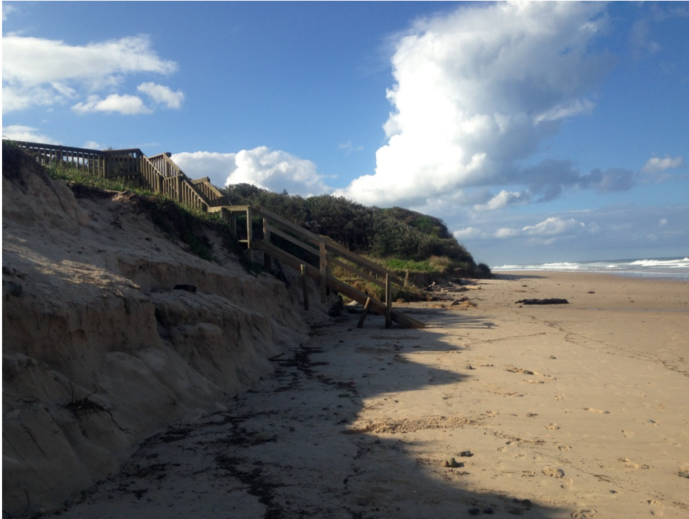
FIGURE 6: EROSION NEAR THE LOOKOUT TO THE NORTH OF THE SURF CLUB, OLD BAR BEACH FOLLOWING THE APRIL STORM. COURTESY OF MICHAEL GRIFFITHS, GREATER TAREE CITY COUNCIL.
