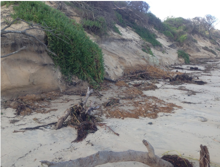
FIGURE 5: ROCK EXPOSED TO THE SOUTH OF THE SURF CLUB AT OLD BAR BEACH FOLLOWING THE APRIL STORM. COURTESY OF MICHAEL GRIFFITHS, GREATER TAREE CITY COUNCIL.
