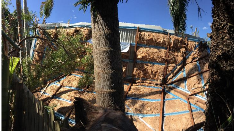
FIGURE 1. WIND-INDUCED FAILURE OF A NEW (< 1 YEAR) METAL CLADDING ROOF ON AN OLD HOUSE AT THE RAFTER TO TOP-PLATE CONNECTION DURING CYCLONE MARCIA (2015) IN YEPPON, AUSTRALIA - THERE APPEARED TO BE NO RETROFITTING OF THE WEAKER CONNECTIONS.
