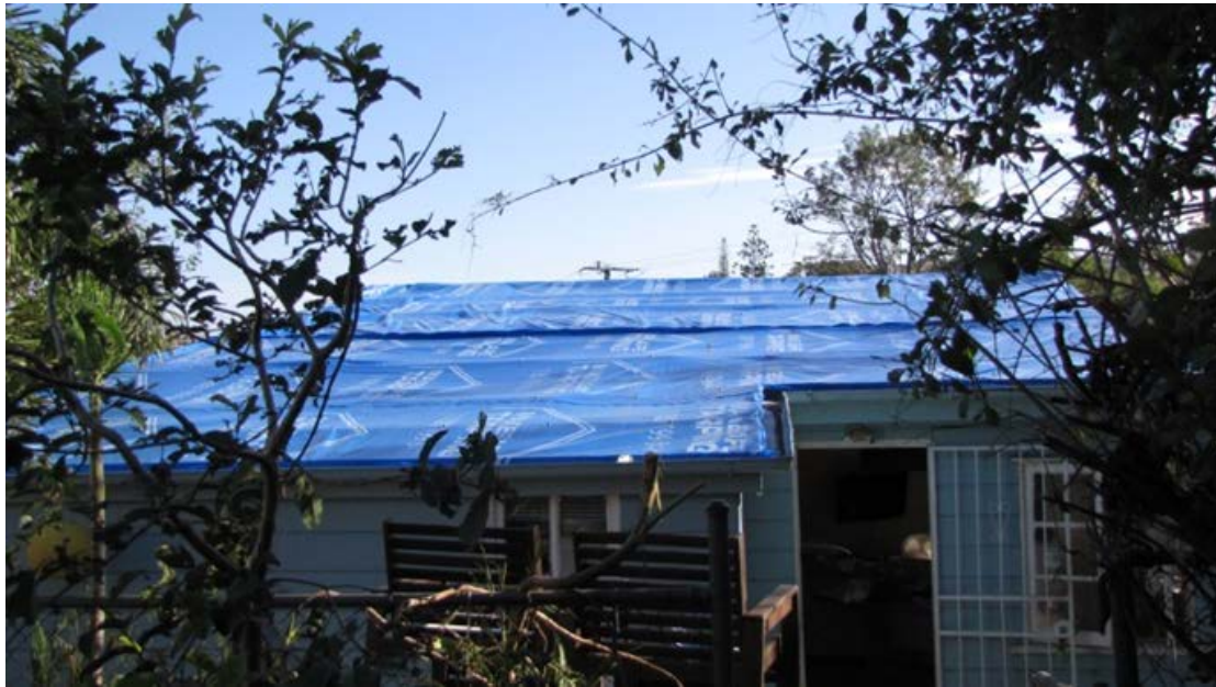
FIGURE 3. FAILED HOUSING AFTER BRISBANE THUNDERSTORMS (NOVEMBER 2014) WITH MISSING ROOFING FROM NOT IMPROVING THE BATTEN TO RAFTER CONNECTION WHEN UPGRADING THE ROOFING TO BATTEN CONNECTION (EXAMPLE 1)
