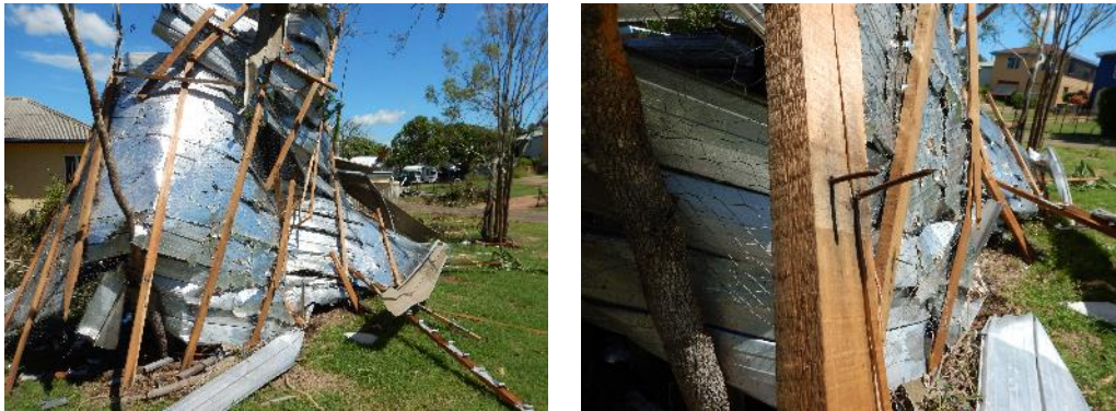
FIGURE 2. WIND-INDUCED FAILURE OF A METAL CLADDING ROOF (LEFT) AT THE BATTEN TO RAFTER CONNECTION (RIGHT) DURING CYCLONE MARCIA (2015) IN YEPPON, AUSTRALIA.
