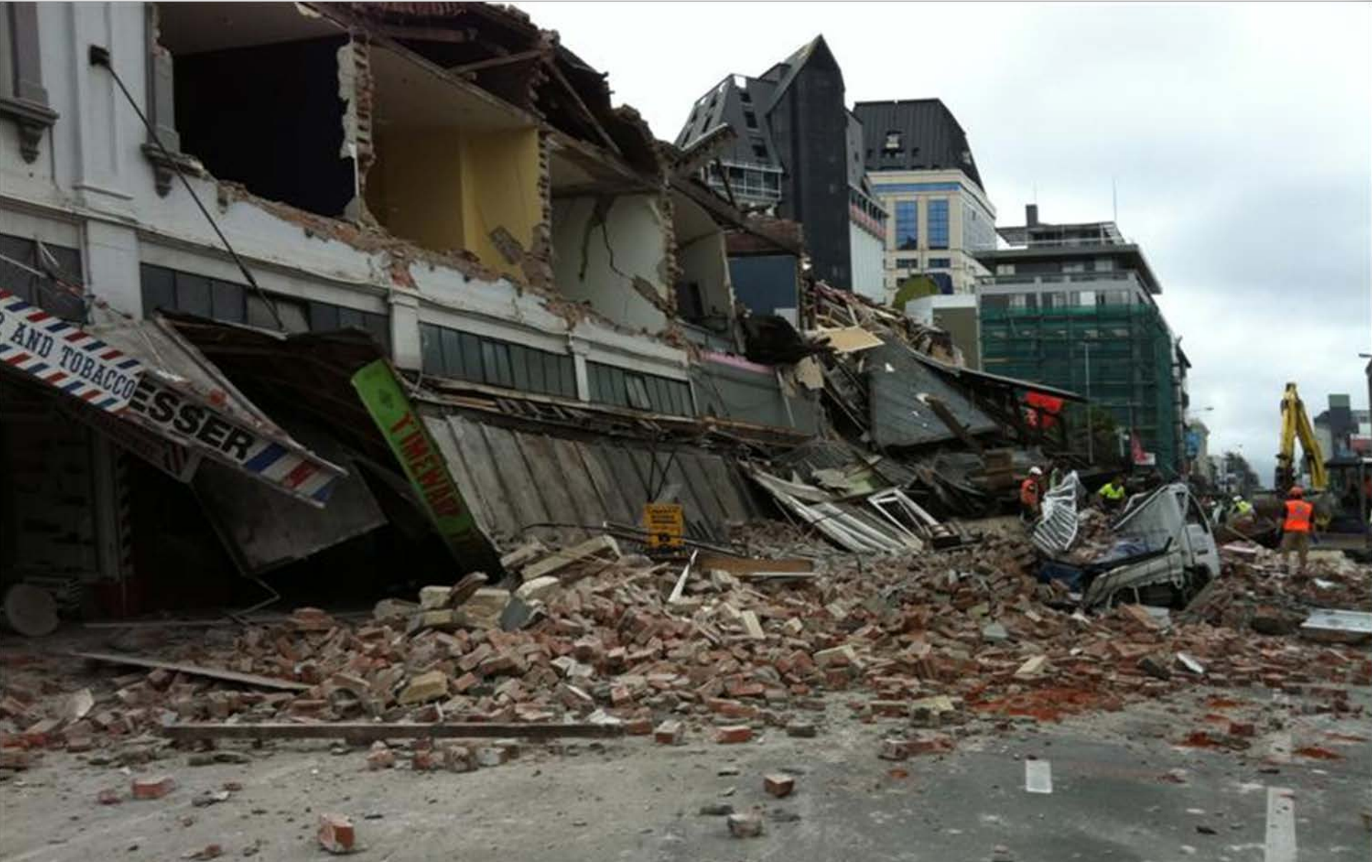
Out-of-plane wall bending failures in Unreinforced Masonry (URM) buildings in Christchurch (42 fatalities)
