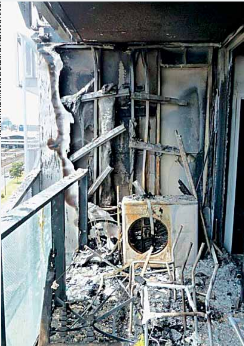
Fire damage on the south wall balcony of apartment 805 of the Lacrosse building.
