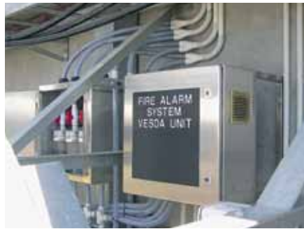
An early warning air-sampling smoke detection system protects a waste recycling facility.
