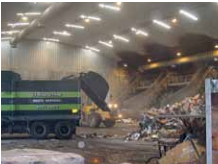
Community waste stations pose significant pollution and contamination challenges for most smoke detection systems.
