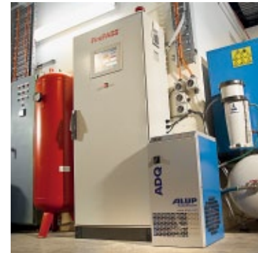
Oxygen-reduction fire prevention system at Sydney Adventist Hospital.
