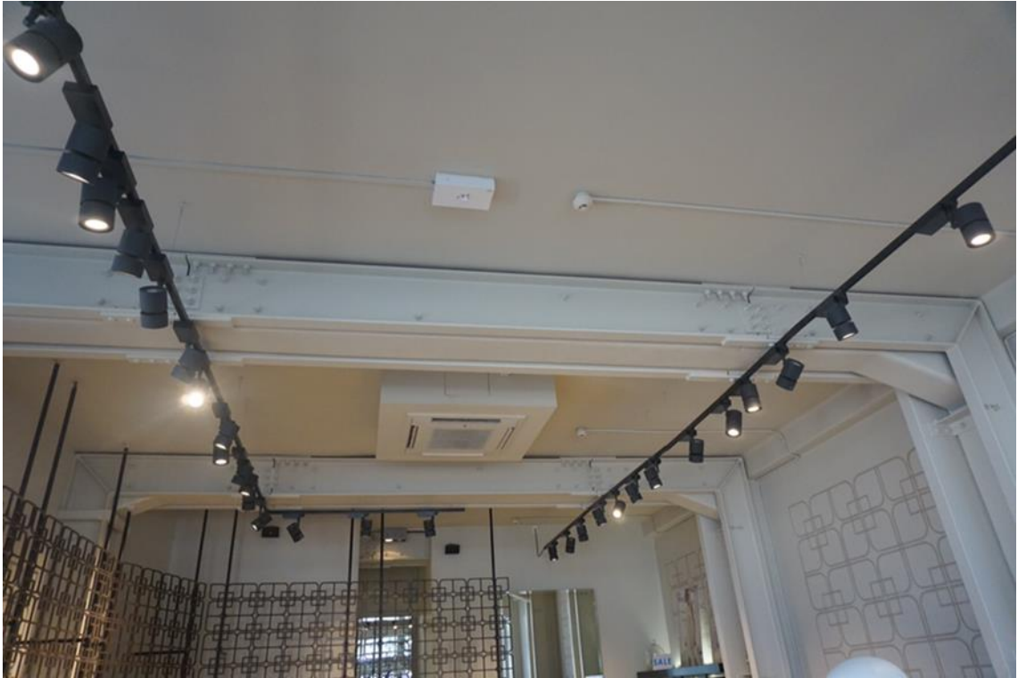
Figure 1: Ground floor view of retrofitted two storey retail structure of the 1930s period in Napier, New Zealand. The building is of poorly detailed reinforced concrete frame construction with unreinforced masonry infill walls. Ductile steel moment frames have been retrofitted to strengthen the structure in the transverse direction.
