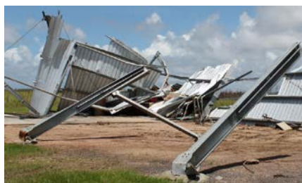
Damage to a shed in Tully from Cyclone Yasi, 2011.
