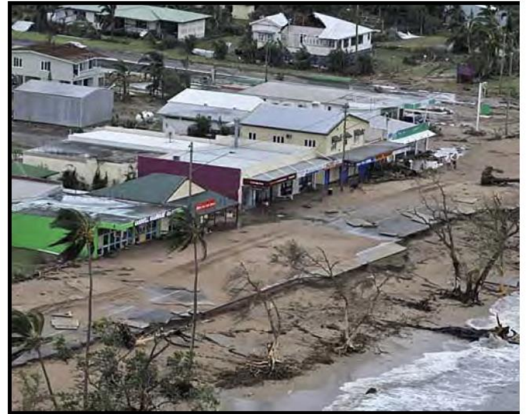
Photograph 31: Coastal erosion and damage to buildings and infrastructure at Cardwell following TC Yasi (Source: News Limited)
