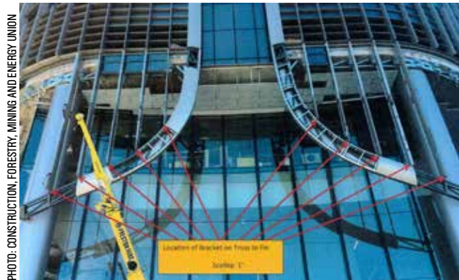
In July this year this new building in Brisbane was found to have been using asbestos-containing gaskets during construction, which were subsequently removed.
