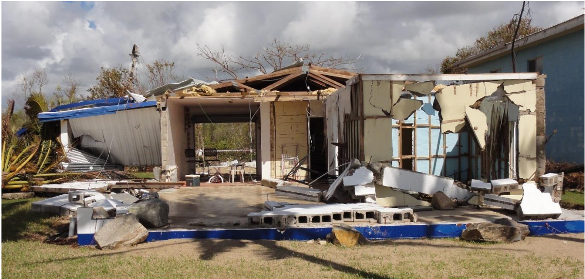
Figure 6. Damage to home caused by storm surge inundation during Tropical Cyclone Yasi.
