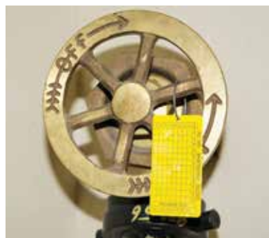
Neglected hydrants can burst on testing.
