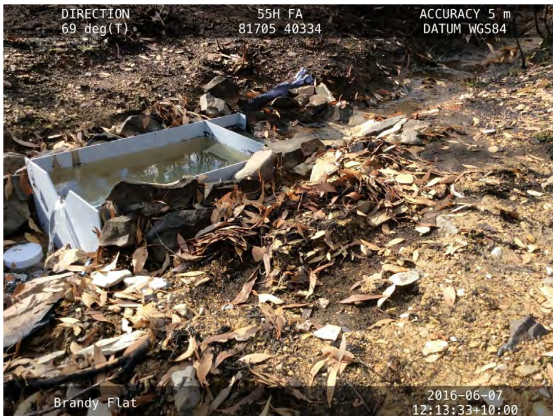
FIGURE 3 - A SEDIMENT TRAP AND A V-NOTCH WEIR INSTALLED IN A BURNED GULLY
