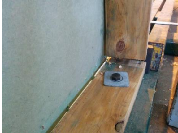
(B) HDF: SHEET FAILURE
