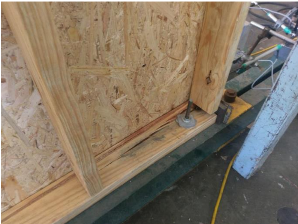
FIGURE B12: OSB BOTTOM PLATE FAILURE (DRY-DRY SAMPLES)
