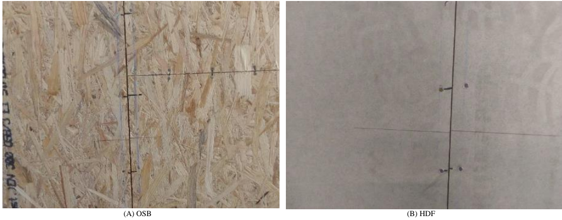
FIGURE B8: SLIPPAGE OBSERVED BETWEEN ADJACENT BRACING SHEETS
