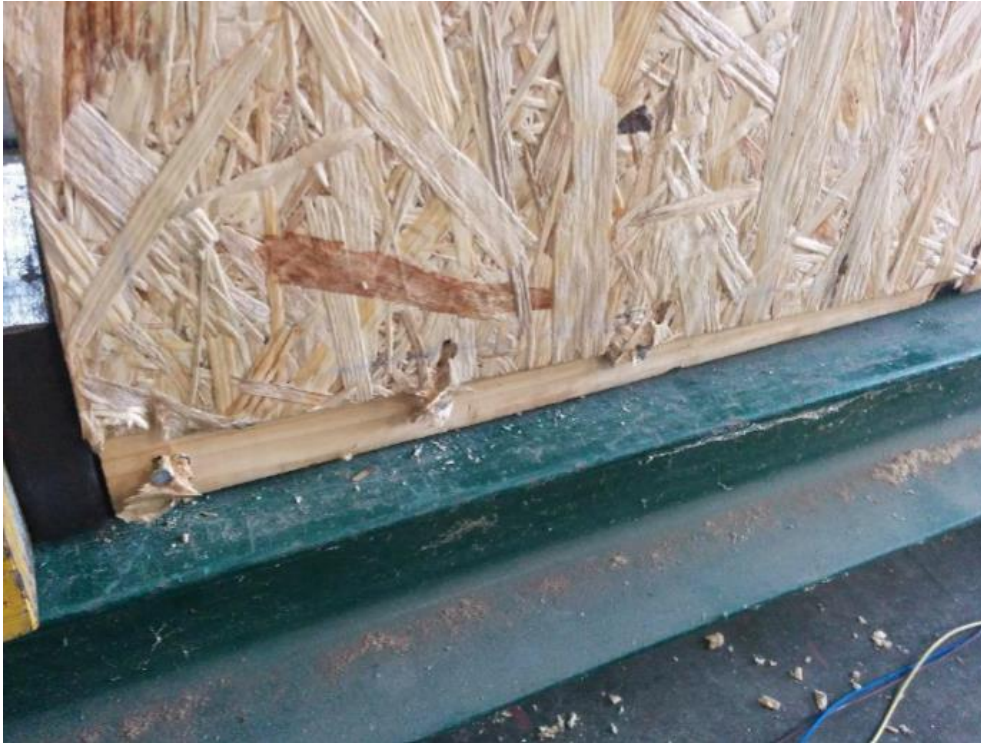
FIGURE B13: OSB BRACE SHEETING FAILURE (WET-DRY SAMPLES)
