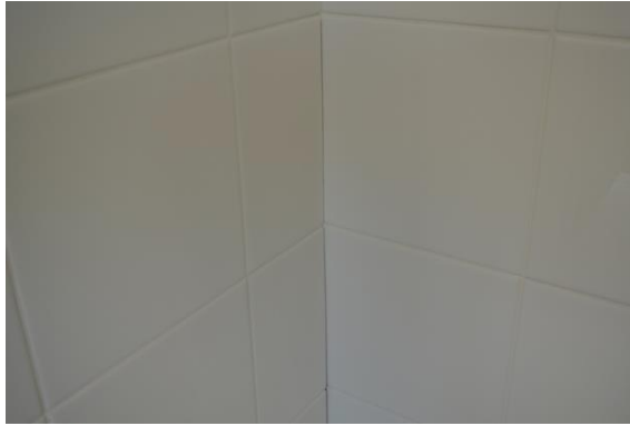
FIGURE 34: GAP BETWEEN TILES AT WALLS CORNERS
