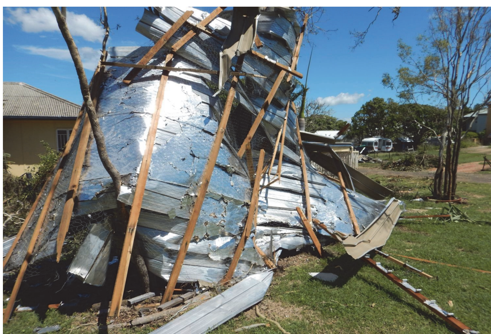
Fig1. Batten to rafter failure caused by Tropical Cyclone Marcia
