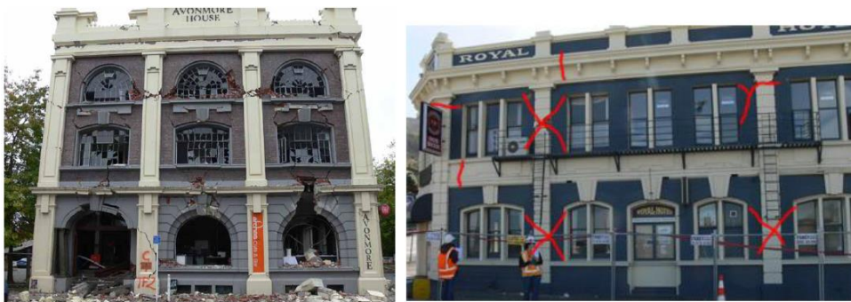
Figure 3: AH and RH building damage
