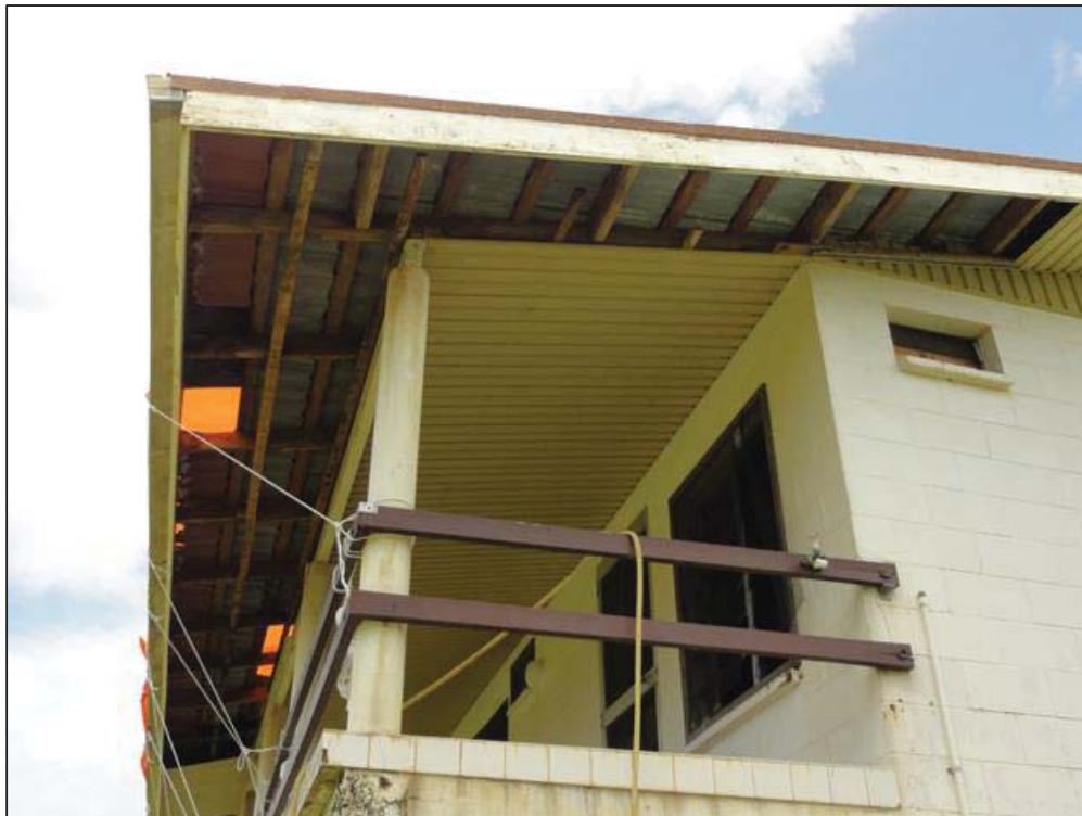
Figure 5: Failure of Soffit, Cyclone Yasi, 2011
