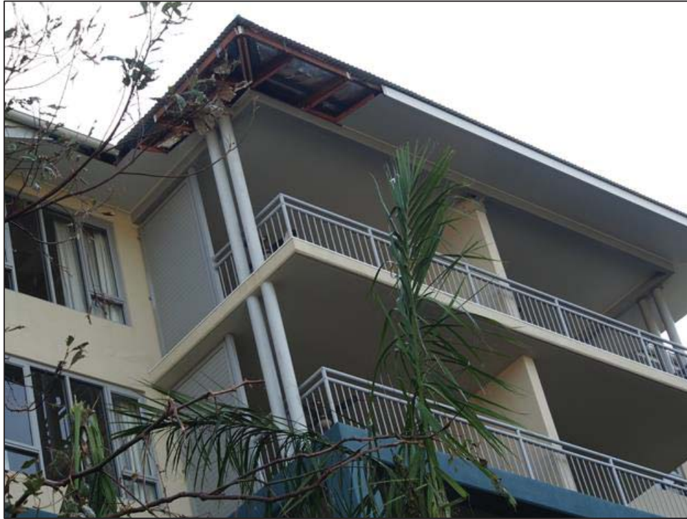
Figure 10: Failure of Soffit, Cyclone Debbie, 2017
