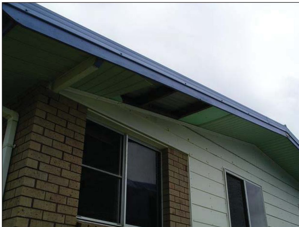
Figure 3: Failure of Soffit, Cyclone Larry, 2006
