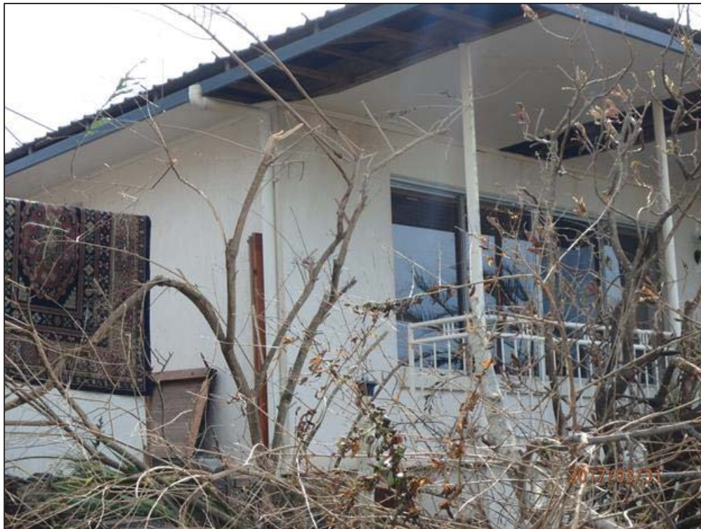
Figure 11: Failure of Soffit, Cyclone Debbie, 2017
