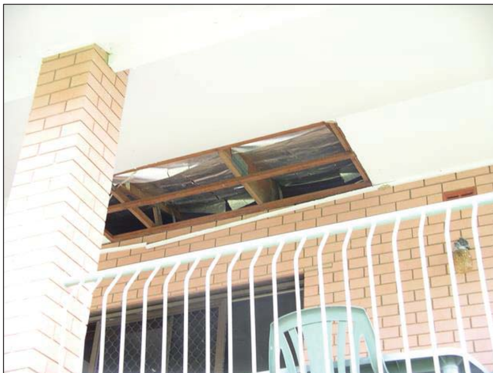
Figure 2: Failure of Soffit, Cyclone Larry, 2006
