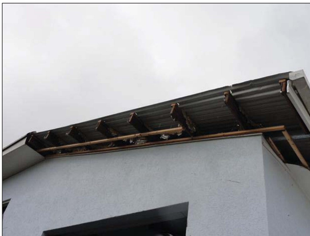
Figure 9: Failure of Soffit, Cyclone Yasi, 2011
