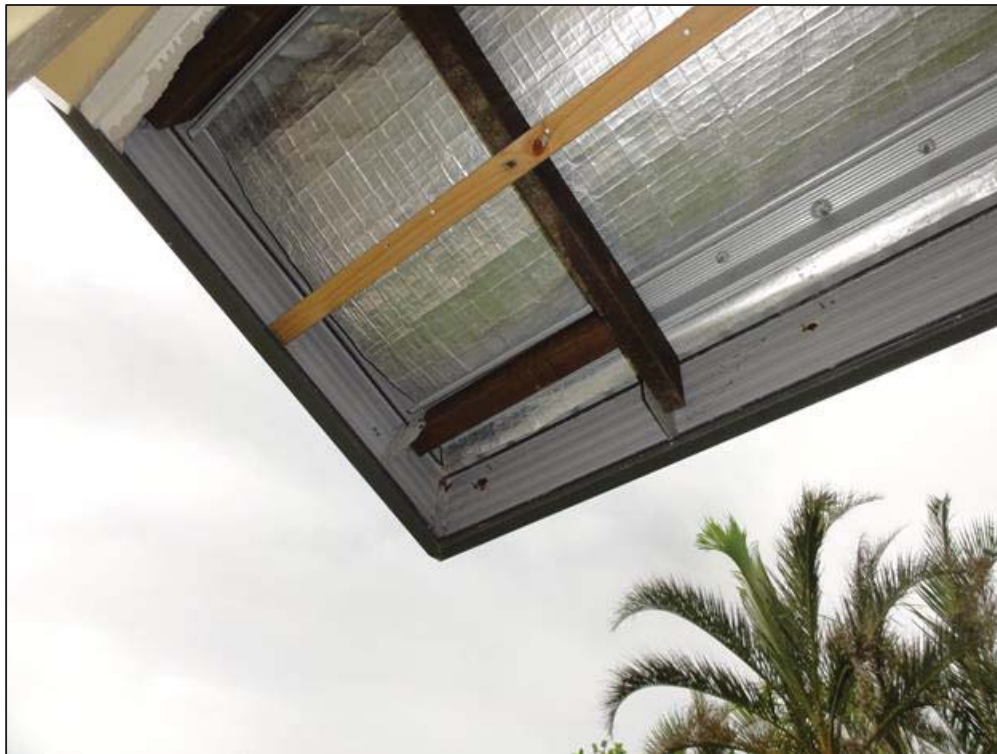
Figure 7: Failure of Soffit, Cyclone Yasi, 2011
