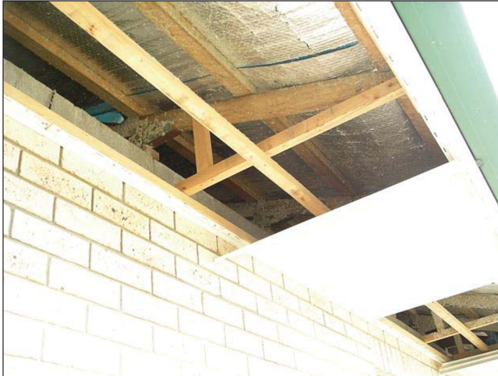
Figure 4: Failure of Soffit, Cyclone Larry, 2006
