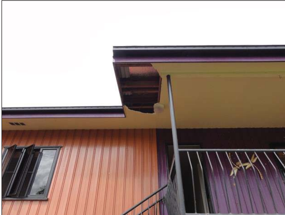
Figure 6: Failure of Soffit, Cyclone Yasi, 2011
