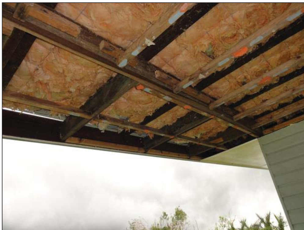
Figure 8: Failure of Soffit, Cyclone Yasi, 2011
