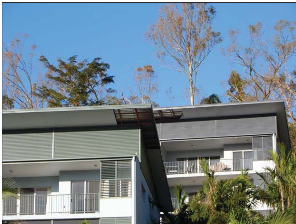
Figure 12: Failure of Soffit, Cyclone Debbie, 2017
