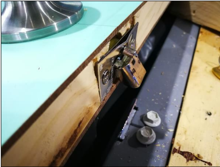
Figure 2. Typical Lock Mechanism Failure
