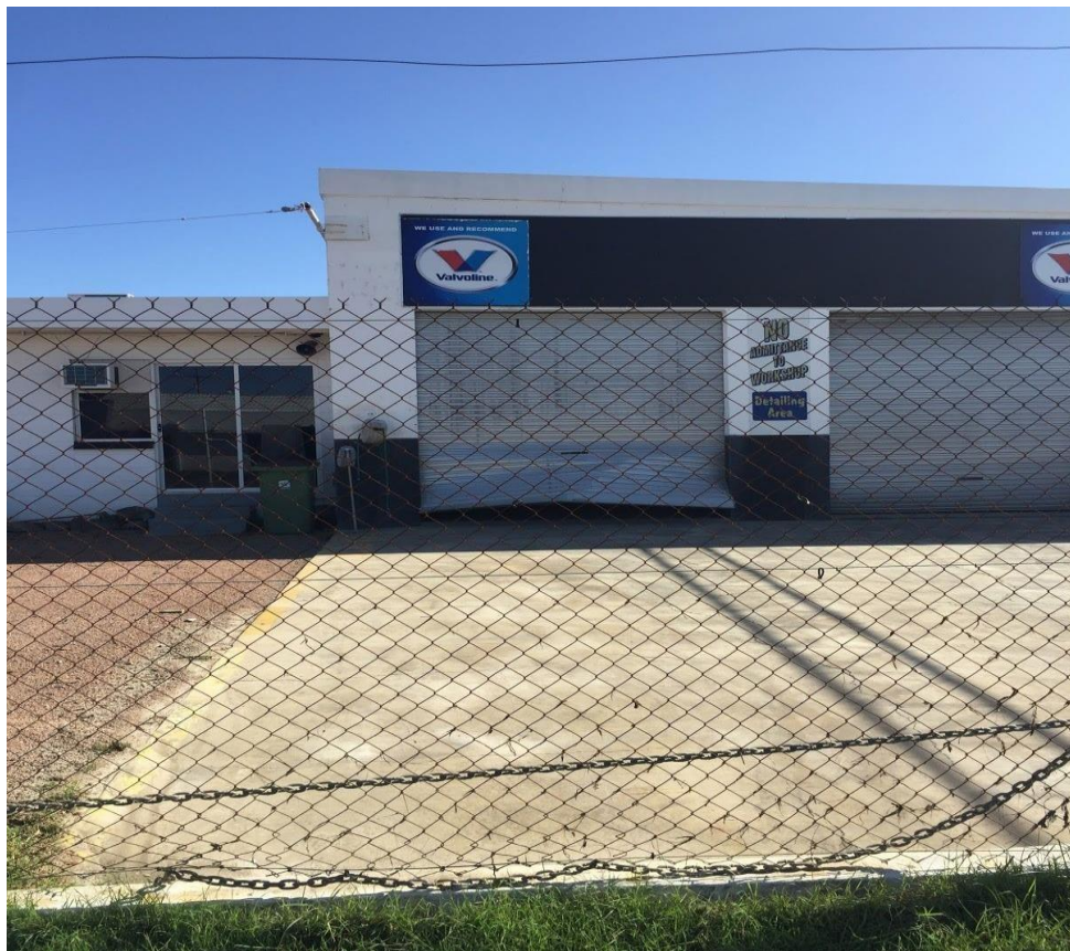
Figure 4 – Showing damage to a commercial property's roller doors in Hyde Park.
