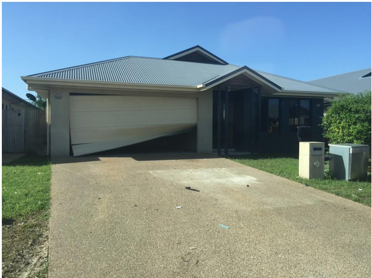
Figure 2: Roller doors in Eastern Idalia potentially damaged by an electrical short. High flow flood waters were ruled out as a cause based on lack of debris and vegetation.
