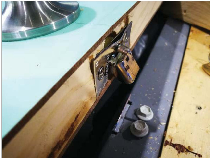
Figure 18: Trial SS5 Broken Lock Mechanism
