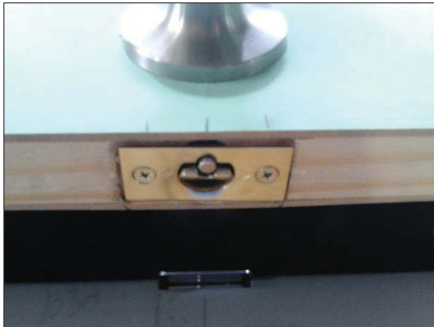
Figure 7: Trial SS2 Lock Jammed
