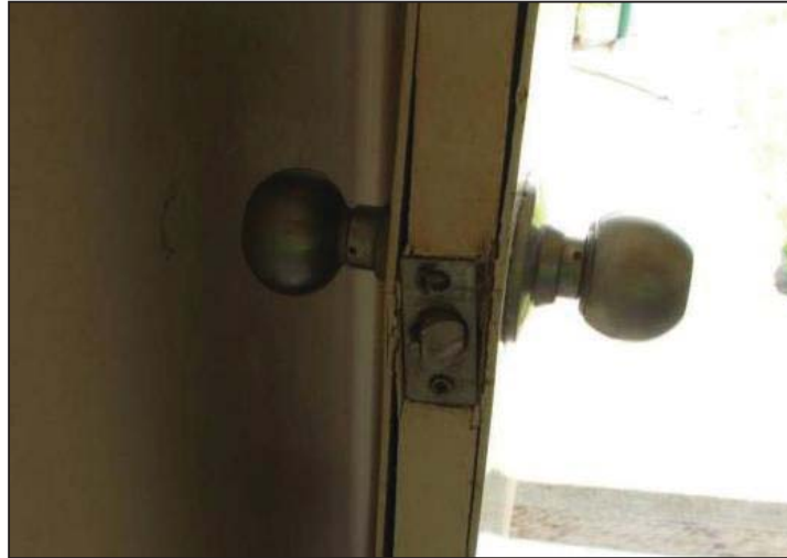
Figure 2: Failure of External Door
