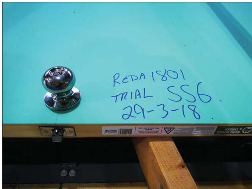
Figure 24: Trial SS6 Damage to Lock Mechanism
