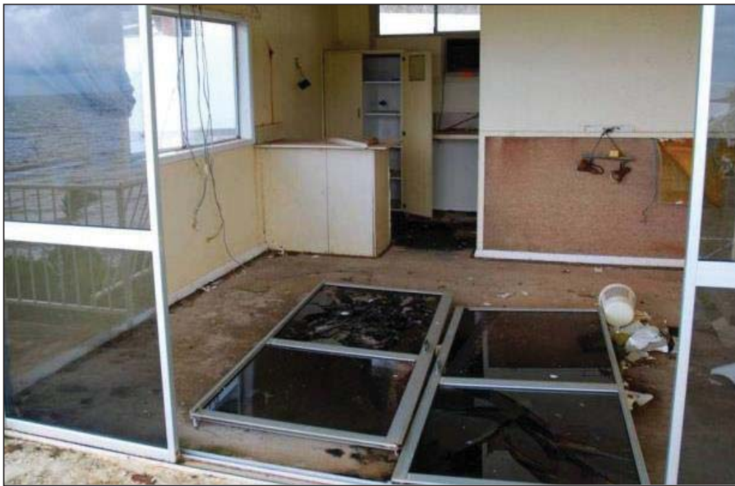
Figure 1: Failure of Glass Sliding Doors
