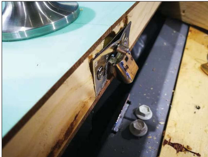
Figure 4: Lock Mechanism Failure
