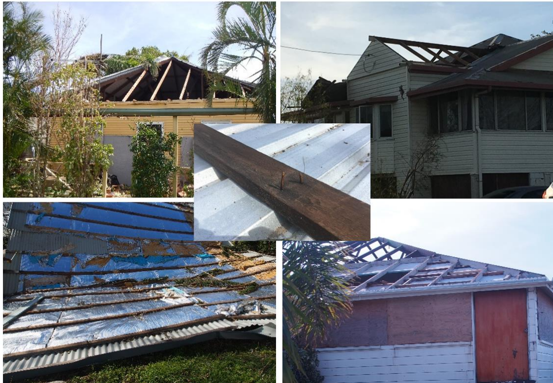
FIGURE 1. WIND-INDUCED FAILURES OF ROOF BATTENS TO RAFTERS ON PRE-80S CONSTRUCTION DURING TC DEBBIE. THERE WERE EXAMPLES OF NEW ROOF CLADDING SCREWED TO BATTENS BUT NO RETROFITTING OF UPGRADED BATTEN TO RAFTER CONNECTIONS (E.G. STRAPS OR SCREWS) WERE OBSERVED.
